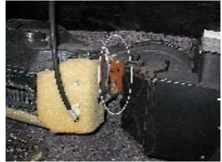
Resistor pack in the heater box
